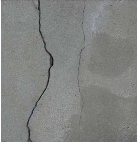
Wear and tear
